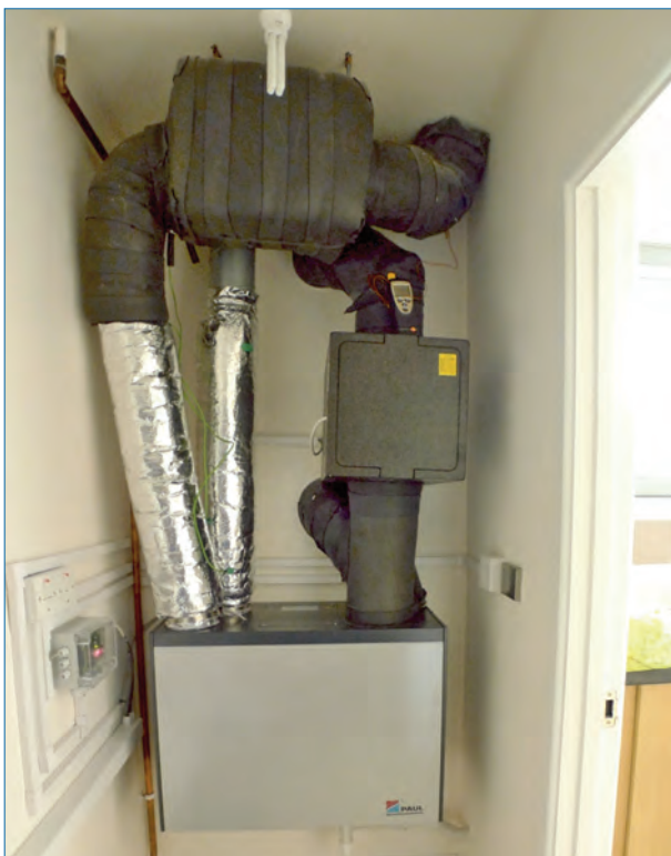
Figure 3: Lime House MVHR
