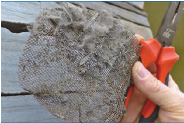
figure 6: Built-in insect screens in the external intake terminals were hard to access and became blocked. The project team removed them and relied on the pre-filters to remove insects.
